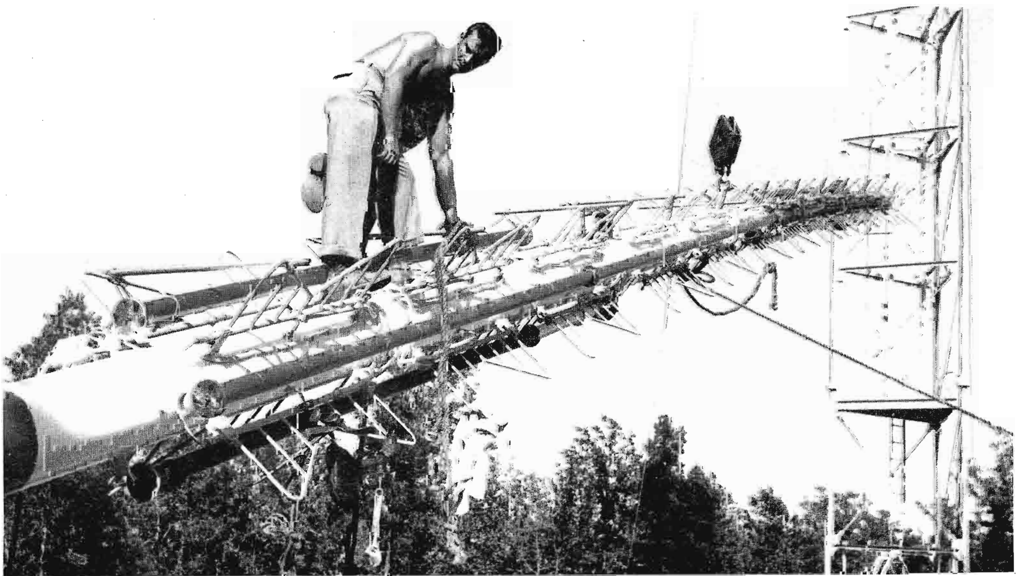
FIG. 12. The TF-12AH superturnstile antenna was raised in one piece to the top of the KSLA 1117-ft tower.
