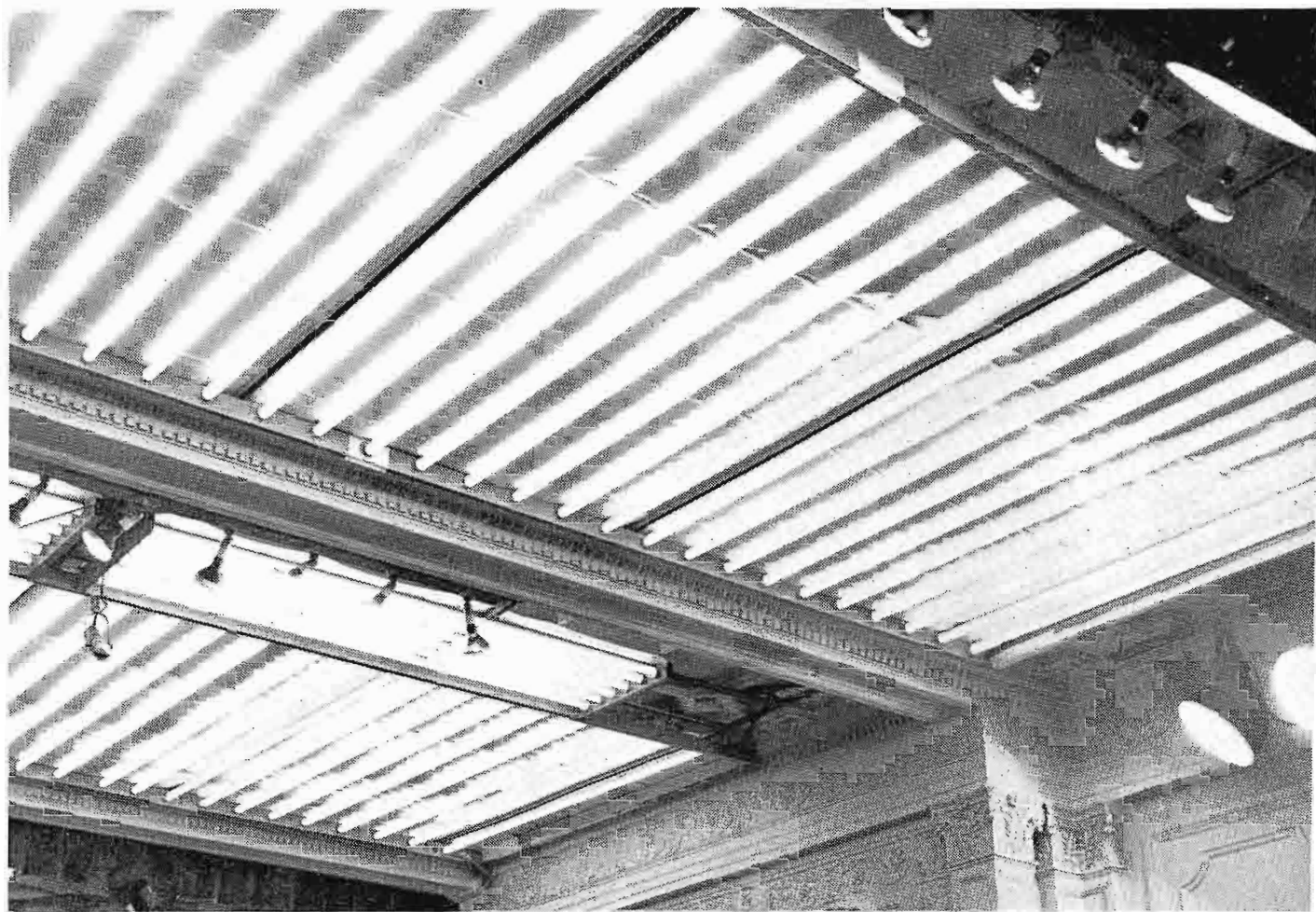
FIG. 22. Partial view of Studio "A" fluorescent lighting banks. Fluorescent lights are used here to provide an even overall lighting for the chapel interior. To get the correct color balance for films, "White" and "Warm White" tubes are used alternately in the lighting sockets.
